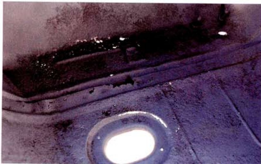
Prior to blasting, the floor seemed quite solid, with little evidence of rust damage. Afterwards, obvious pinholes were found in the driver-side floor and drain hole, requiring future work.
