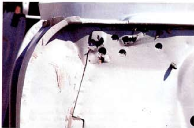
Blasting revealed the full extent of the damage. The repair must be accomplished while maintaining OE bracing and bolt-hole location.
