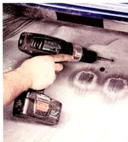
An existing hole in the trunk is used for running the front and rear airlines. Matt enlarges the hole slightly to make room for the lines.
