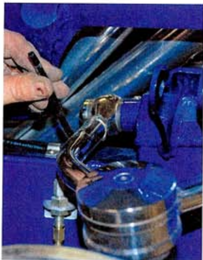
The air line is run through the firewall along the framerrails and cut to length.
