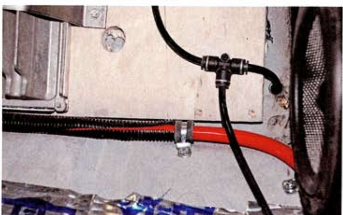
The air lines are run through the interior and split at the T-fitting mounted on the interior firewall.
